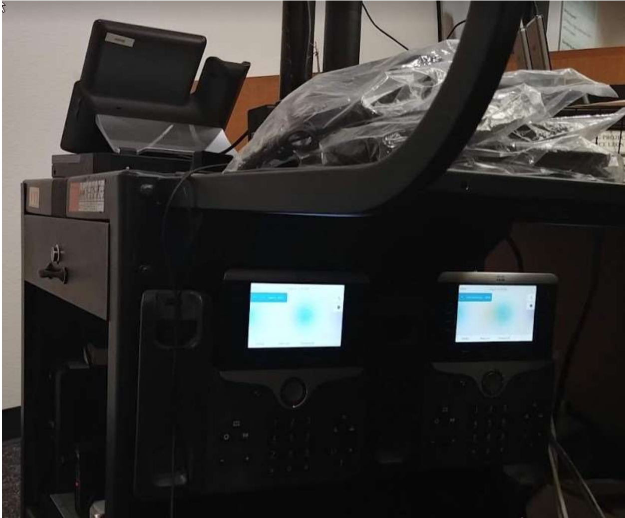
View of Cisco phones. Three phones were used for courtroom operations. One is connected to the dome, one is connected to wireless headsets and one is connected to wireless headset transmitter/receivers. The wireless transmitter/receivers would be used for private conversations. Interpreter station has ability to call each phone separately.
