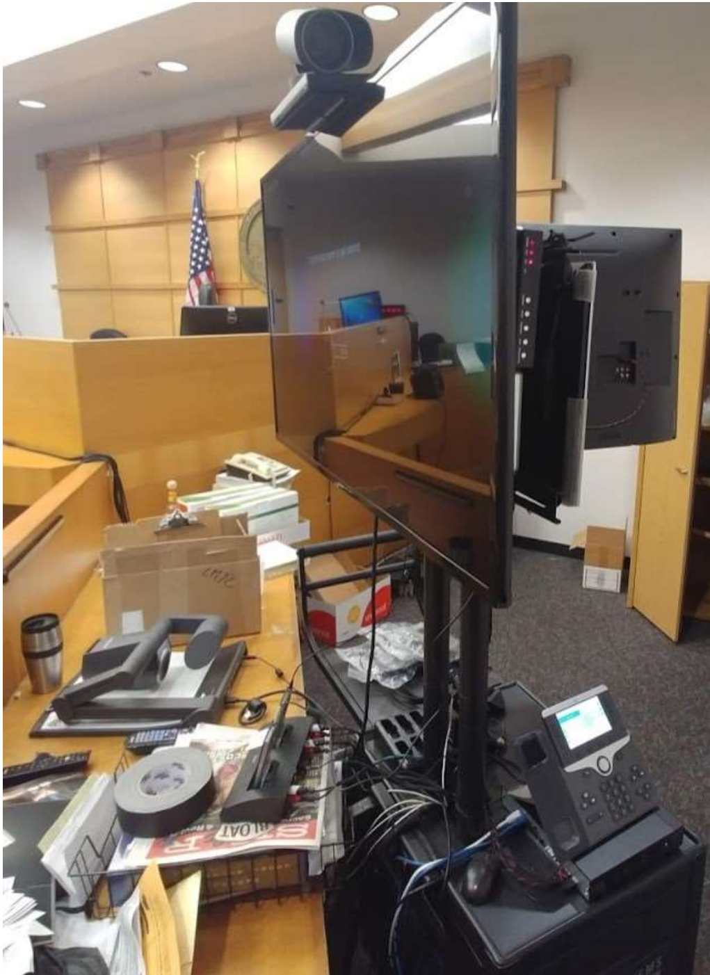
Side view of media cart. Equipment from left to right: document viewer on counter, wireless headsets in charging stations, camera for SX20, courtroom monitor, video converter, SX20, second monitor, and Cisco phone.
