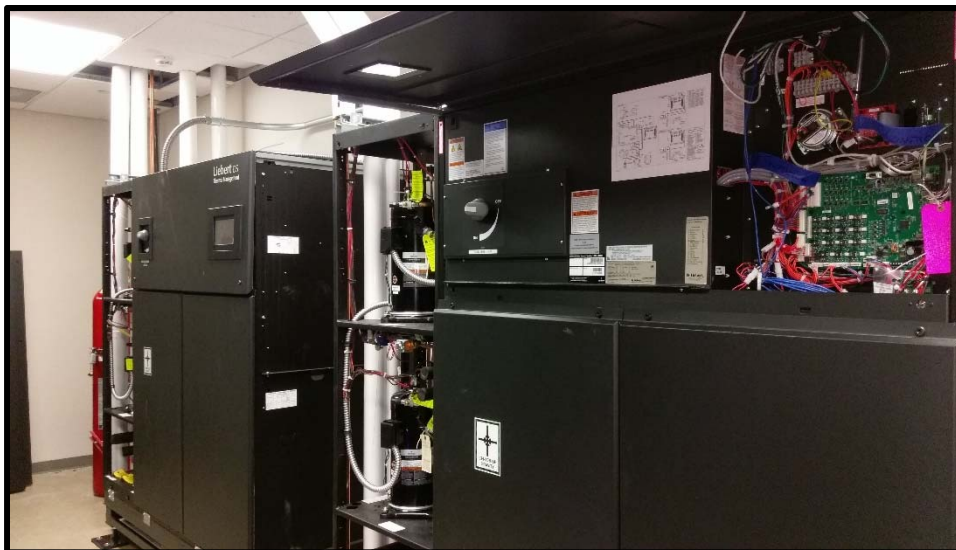
Above: Tuning up by making final adjustments to the units. Below: New rooftop condensing unit.
