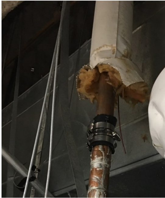
Old failing pipe repair no longer stopping water flow
