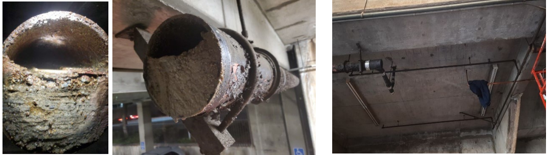
Planter drain lines obstructed with cement
