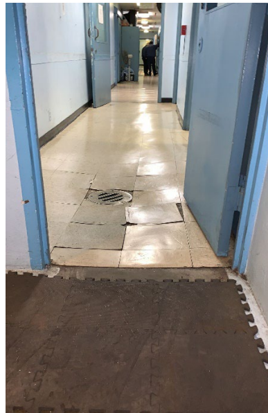
Damaged floor tiles lifting resulting in a safety hazard.
