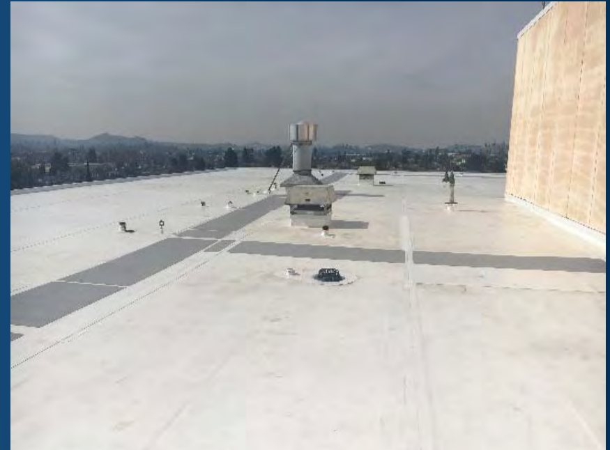
AFTER: Newly replaced roof with Class-A fire rated, 80 mil PVC, Single-ply membrane.
