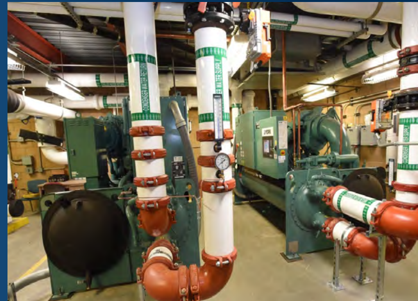
AFTER: Two newly replaced 250-ton magnetic bearing chillers.
