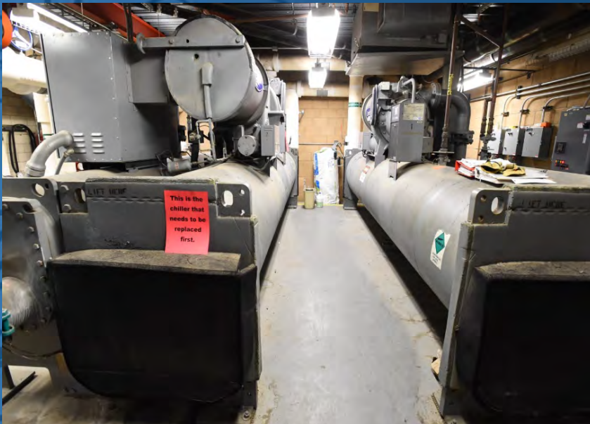
BEFORE: Two failing chillers at Larson Justice Center.
