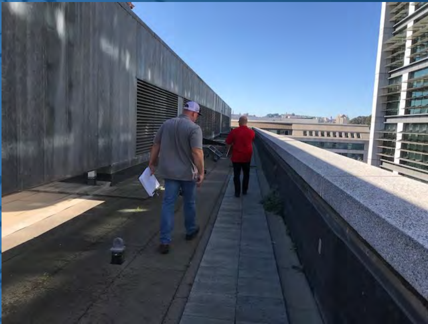
BEFORE: Old failing roof at Civic Center Courthouse.
