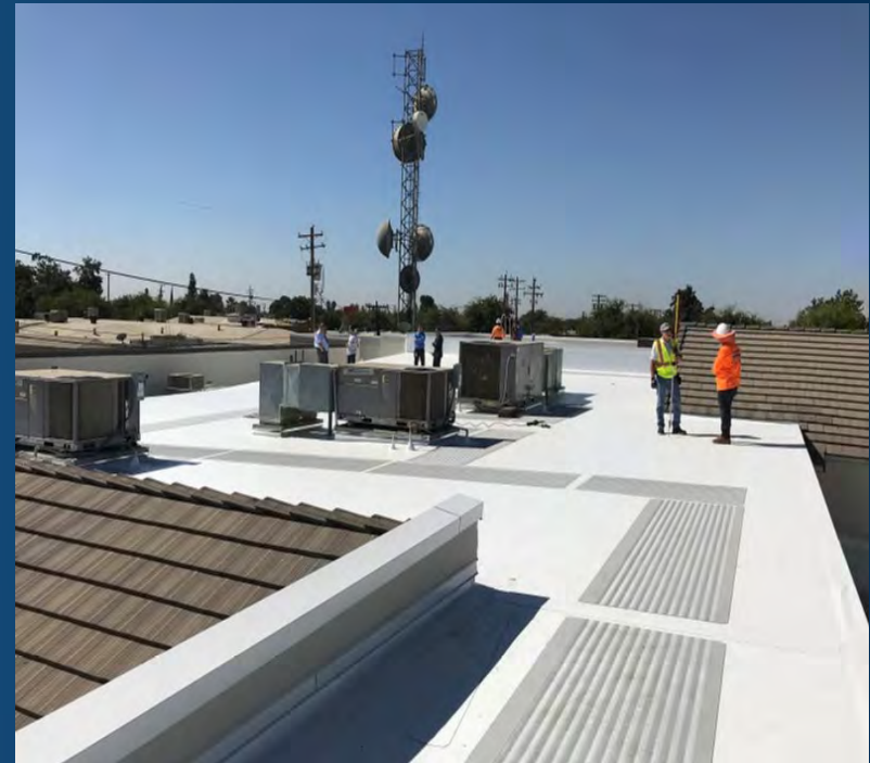
AFTER: Newly replaced roof with Class-A fire rated, 80 mil PVC, Single-ply membrane.
